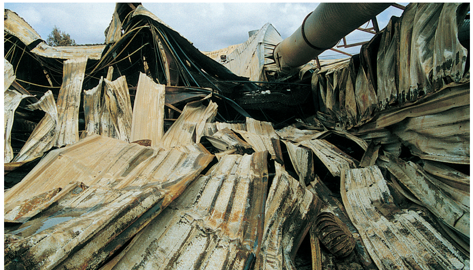
Failure to properly manage hot work can result in a catastrophic fire.
